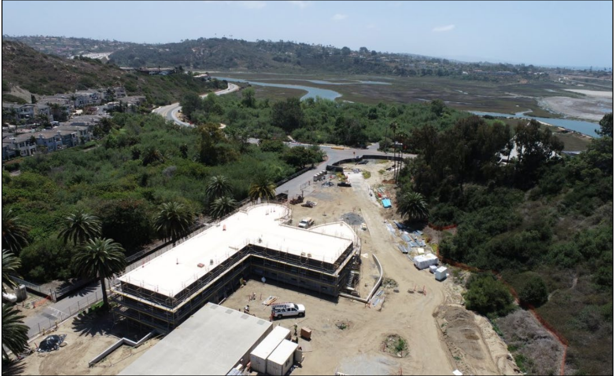
Construction of the new operations and administration building at the San Elijo Water Campus.
