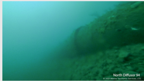
North Diffuser 94 © 2021 Marine Technomic Services, LTD.
