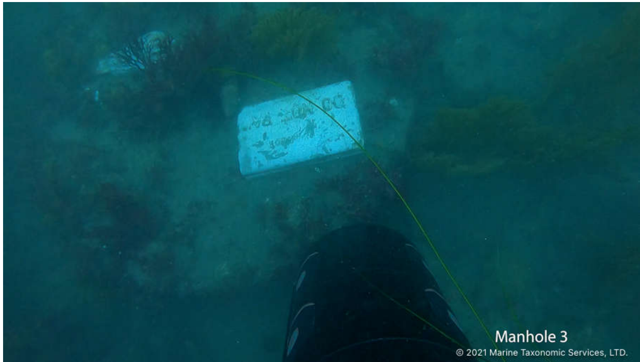
Figure 3. Porthole 3 cover with zinc anode with approximately 50% remaining life expectancy.
