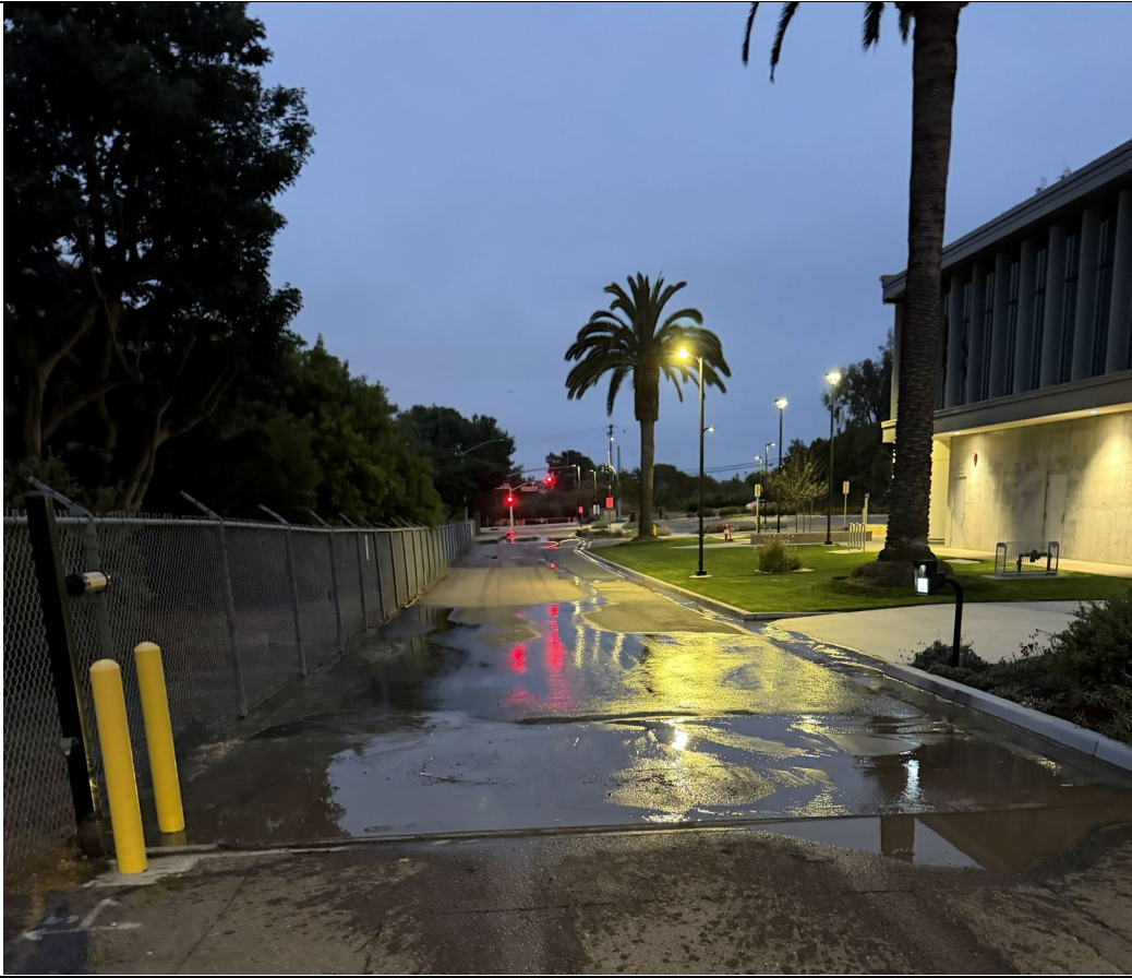
May 8, 2026 Leak Observed at East Entry Gate
