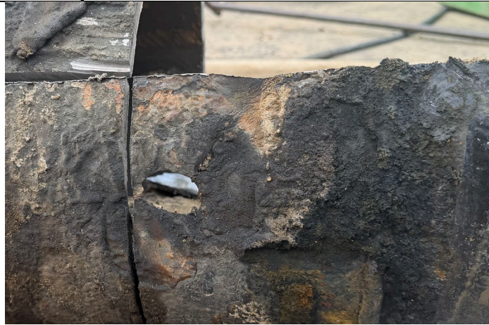
May 8, 2026 Hole in exterior of 12" ductile iron pipe
