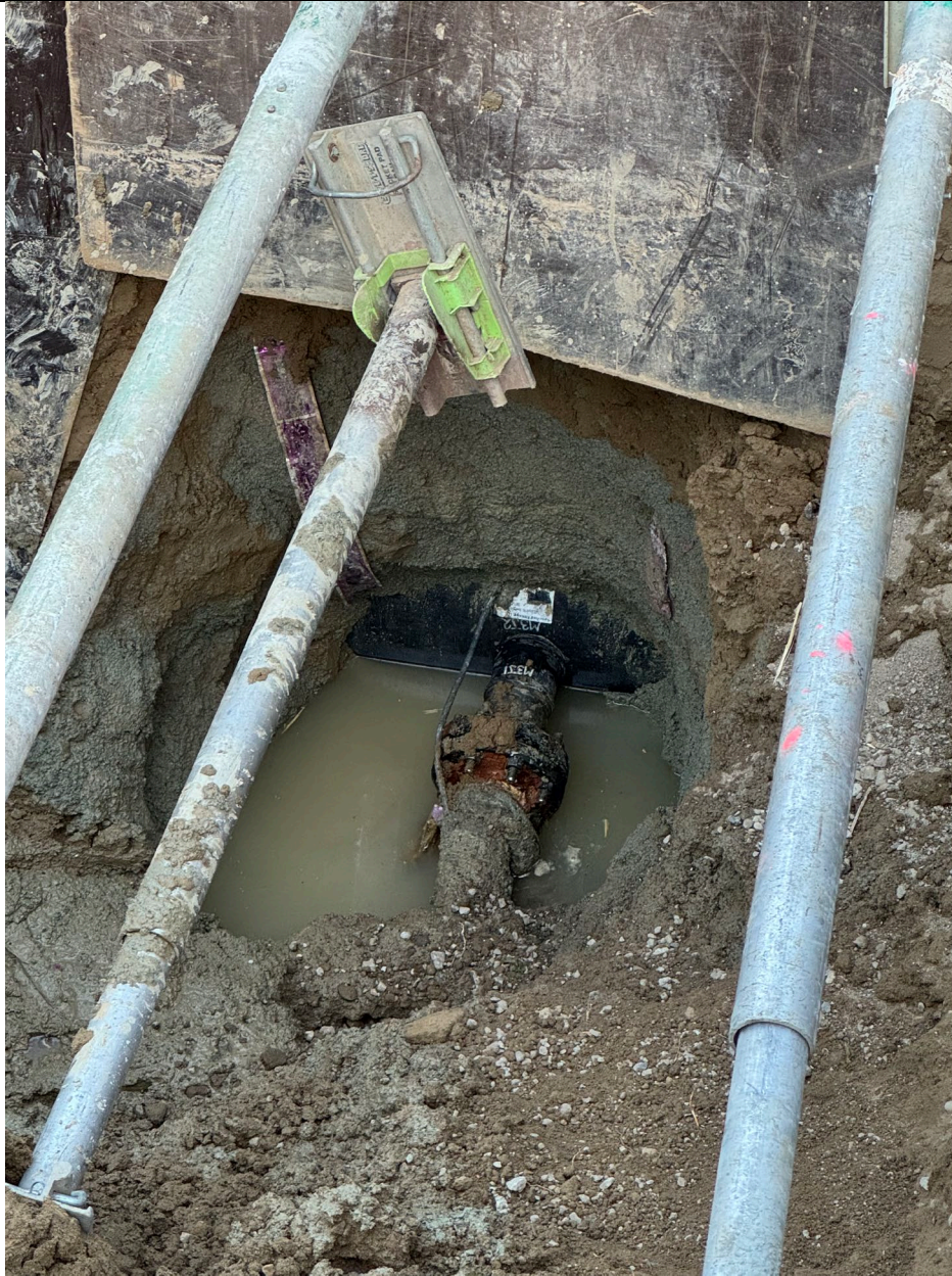
May 18, 2026 Failed Fitting on HDPE (Blowoff Connection)
