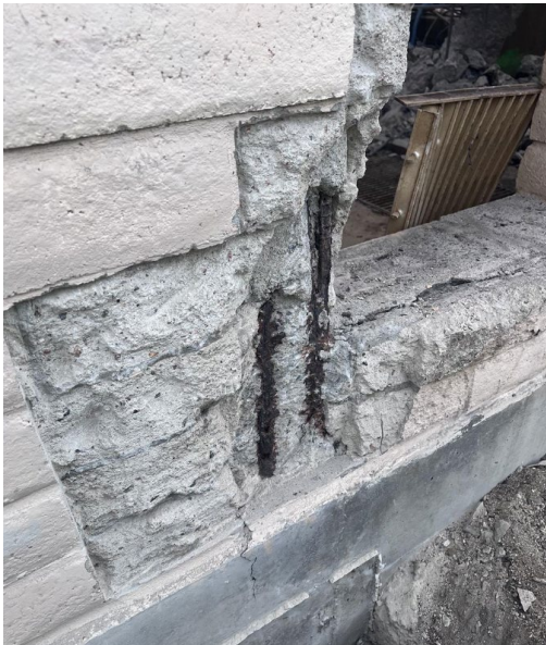
Photo 1 – Example of deteriorated masonry and corroded rebar at wall opening
