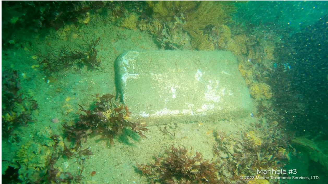
Figure 3. Porthole 3 cover with zinc anode with approximately 50% remaining life expectancy.
